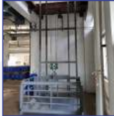
(D-2) HOIST TYPE GOODS LIFT
